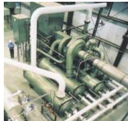
One 10,000 HP (7455 KW) MSG® Air Compressor installed at an air separation facility. One 11,000 HP (8200 KW) MSG® combination Nitrogen Feed/Recycle Compressor is also installed.
